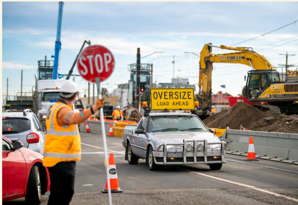
Traffic management located on Nepean Highway in Edithvale to help safely coordinate traffic and manage truck movements
